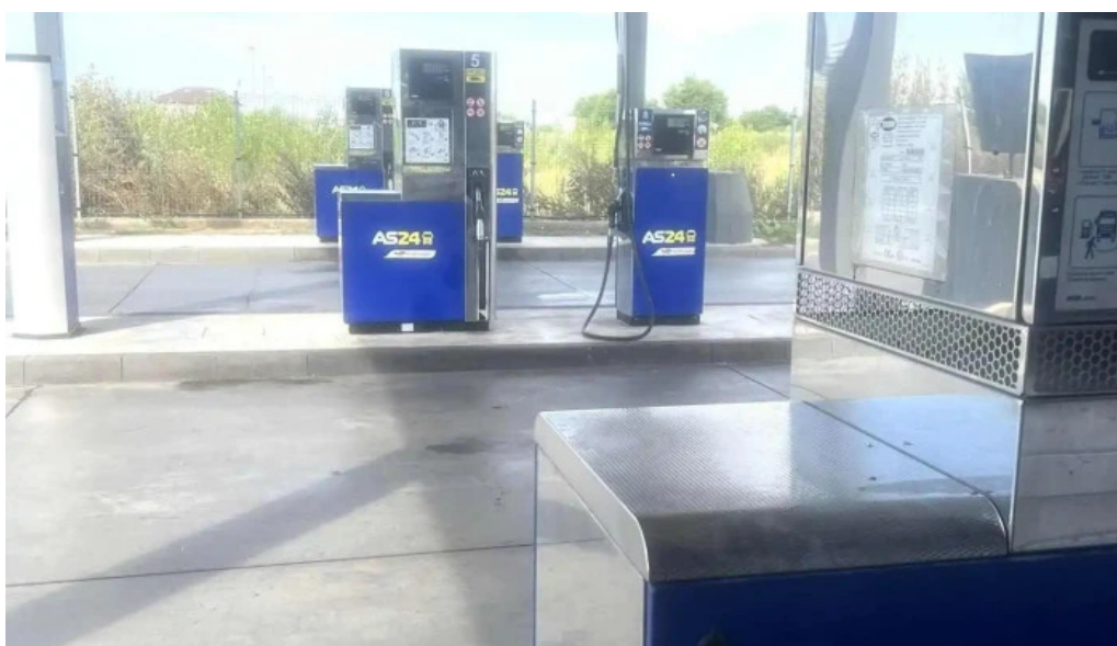
As 24 pompa de combustibil
